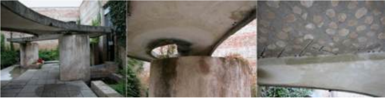
Figure 1. The effects of the passing of time in reinforced concrete elements of Giardino delle Sculture in Biennale Italian Pavillon
