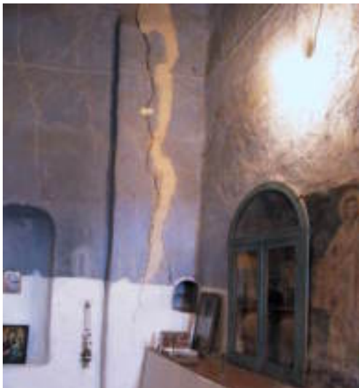
Figure 3. Particular of the monastery interior with a notable fissure in evidence.
