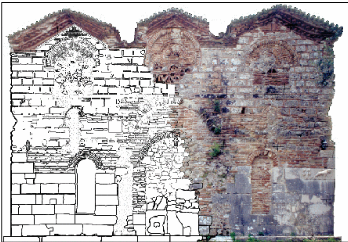
Figure 8. Photoplan of the monastery west facade with a partial vector drawing (reduction from 1:50 scale plot).
