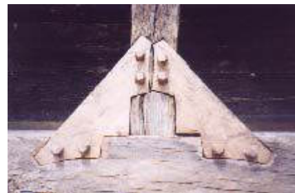
Wooden nails, used for the fixing of the pillars to the foundation
