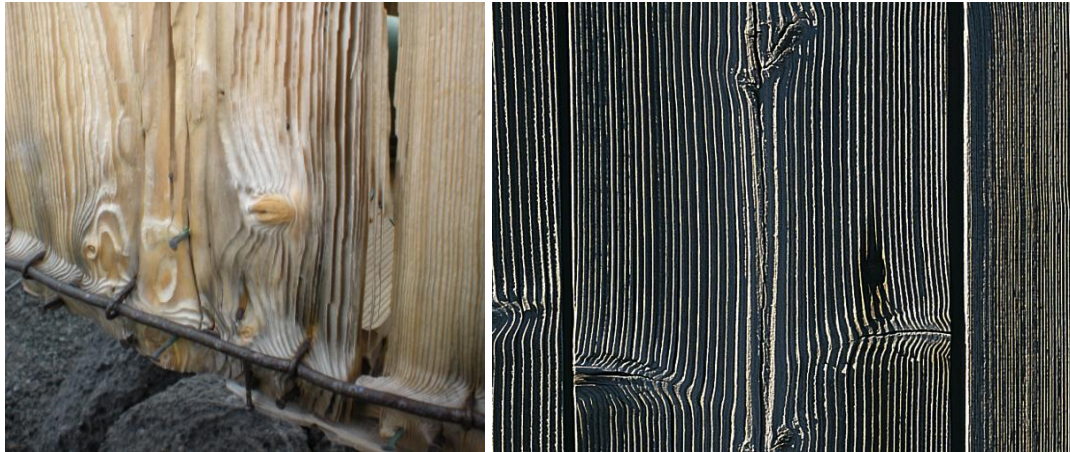
Figure 3: Differential ablation on exterior timbers.
