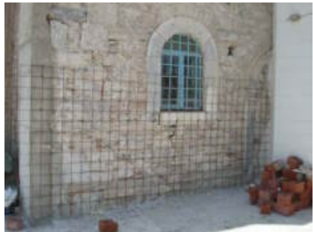
Figure 6. The traces of the church's entrance behind the minaret, documented during the strengthening in 2004.
