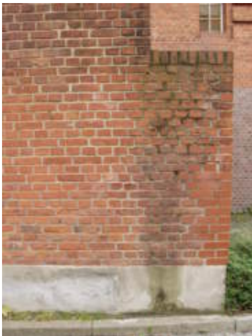
Figure 1. Test object: Masonry affected by moisture and biological cover
