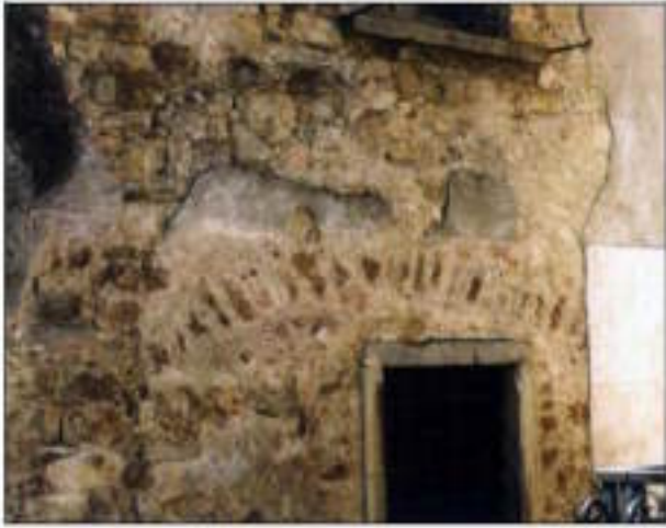
Image 12: To reinforce the masonry usually curb stones or bricks were used to create façade arches
