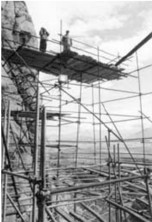
Figure.4:the semi-hanged scaffolding as the station for geodetic works at about 80 meter high
